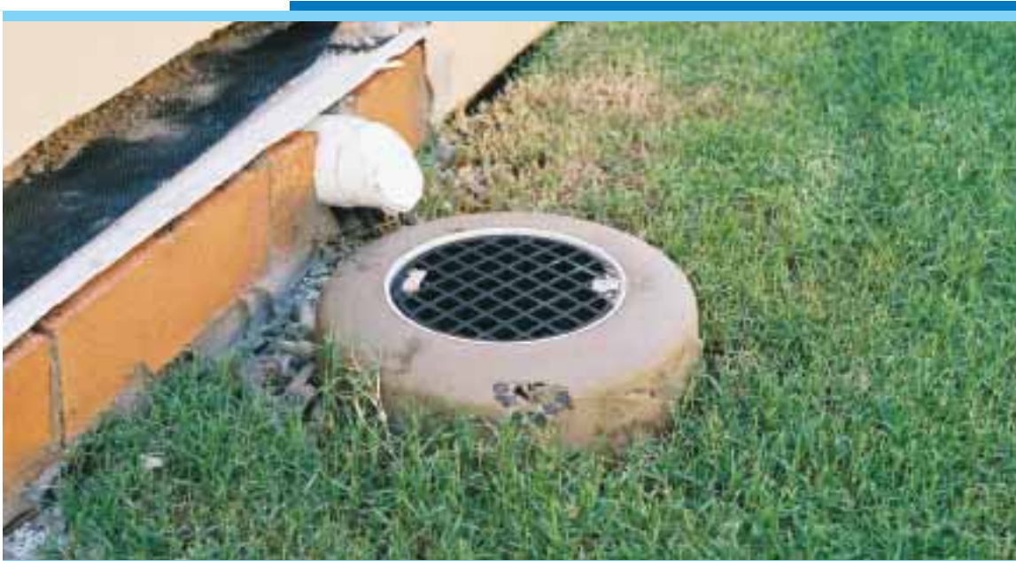
Above: Example of raised overflow relief gully (ORG)
